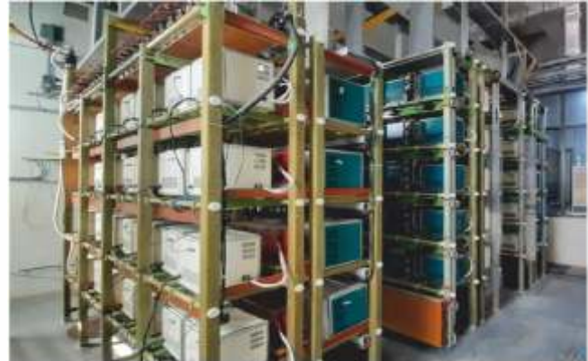
Two DC power supplies of ratings -11kV, 35A & 35kV, 15A are developed and are in operation at the Institute for Plasma Research (IPR) since 2015.
