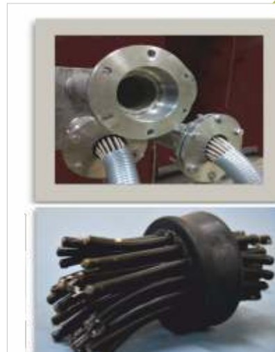
Leak tight feed through flange installed in a hot cell at IGCAR
