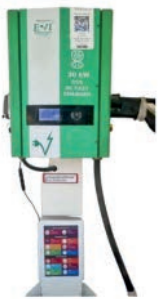
CCS EV AC Fast (Type 2) Chargers by DRIIV Cluster of OPSA
